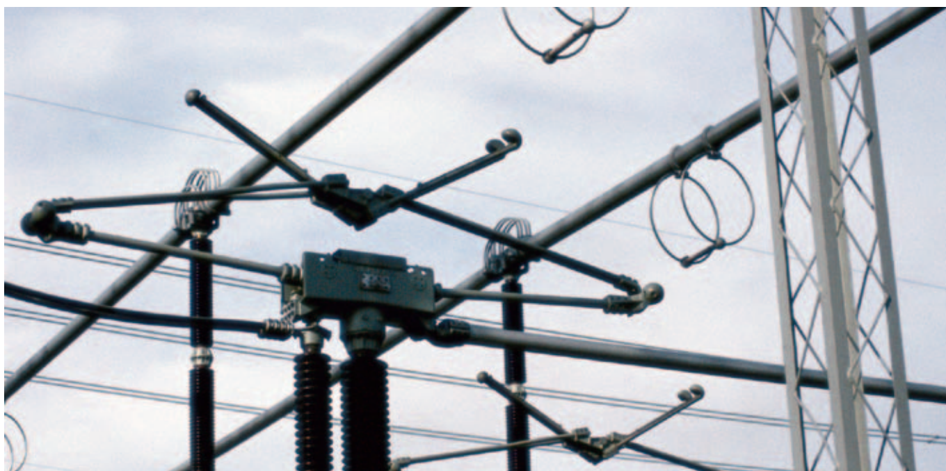
E.ON is a world-leading electricity and gas company operating at all value adding levels from the production and supply through to distribution. The picture shows a transformer station within the electricity transmission.
